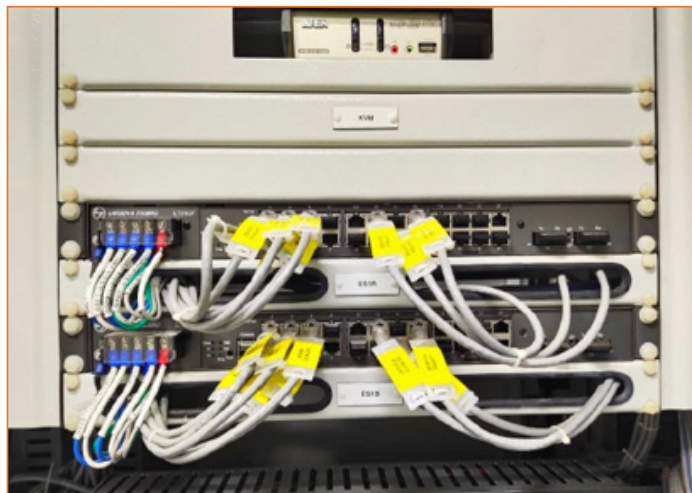
i5Com iES26GF's wired and connected in cabinet bays ready for pre-testing.
