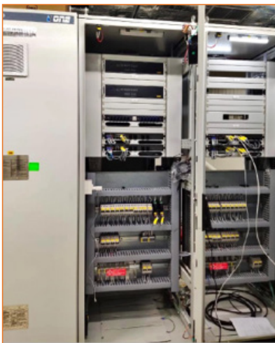
i5Com iES26GF's mounted in cabinet bays.
